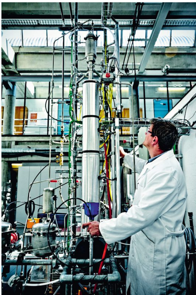
Fig. 3. Distillation unit heated by solar thermal energy.
